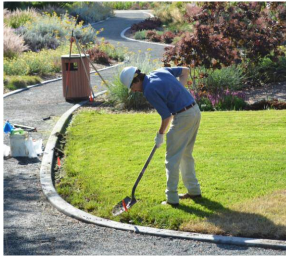
3. Remove a 12" wide strip of the lawn down 3" below the adjacent pavement.
