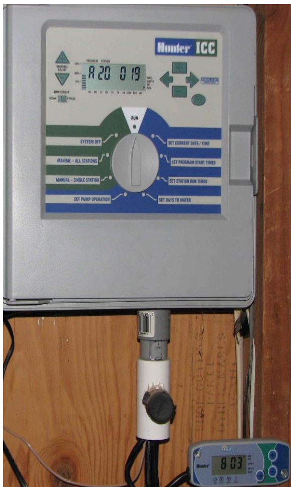
Figure 2 Hunter ICC Controller & SolarSync (Lower Right)
